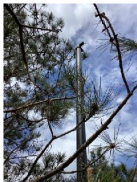
Clubhouse lot Lighting
